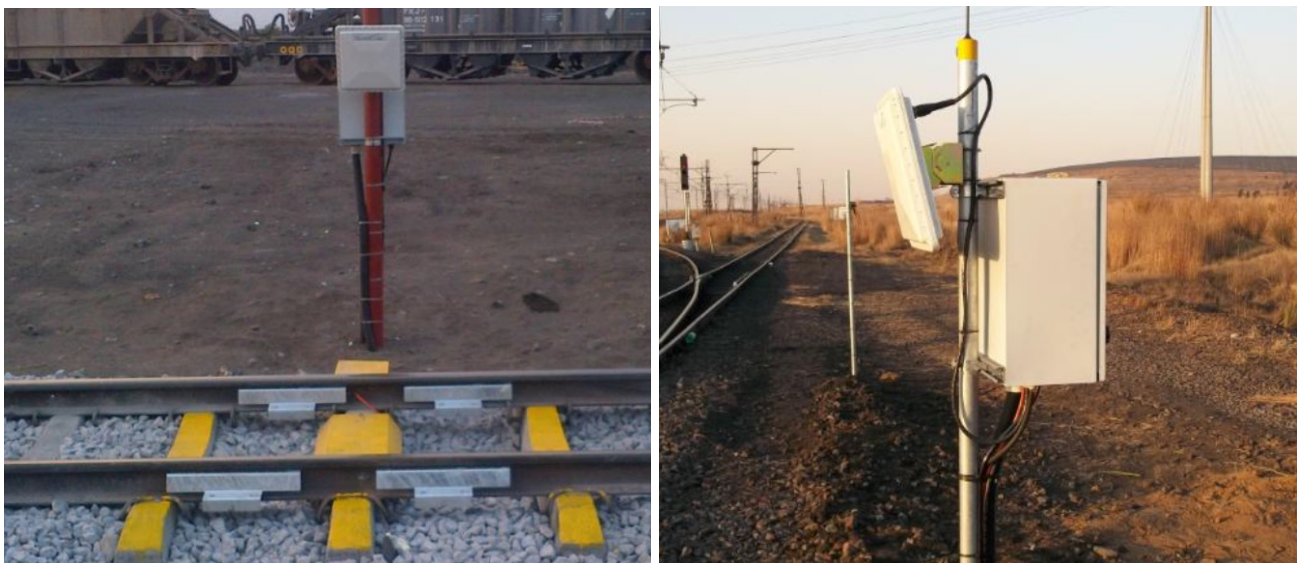
Figure 1 – Typical in-motion weighbridge installation
