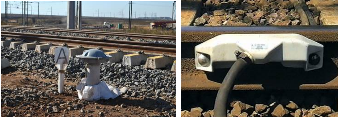
Figure 9 – Example of track vacancy detection equipment
