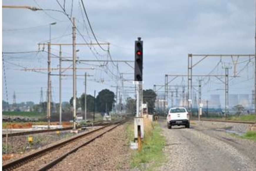
Figure 7 – Example of a typical multi-aspect colour light signal
